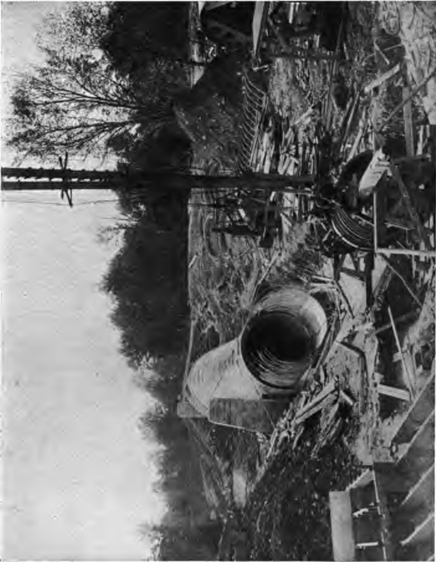
PLATE 171. —Venturi Meter in Construction. Bronze Throat Casting being Set. Portion under Pressure Reinforced. This meter will record the full flow of the cut-and-cover aqueduct. There are three of this type above the city line and one in City Aqueduct Tunnel.
